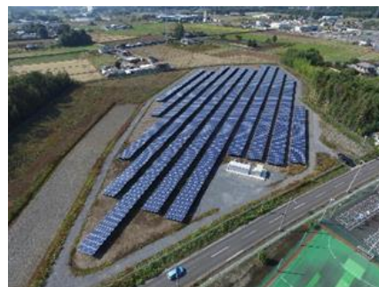
Haru Mito Solar Power Plant
