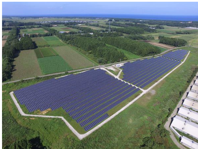
Misawa Solar Power Plant
