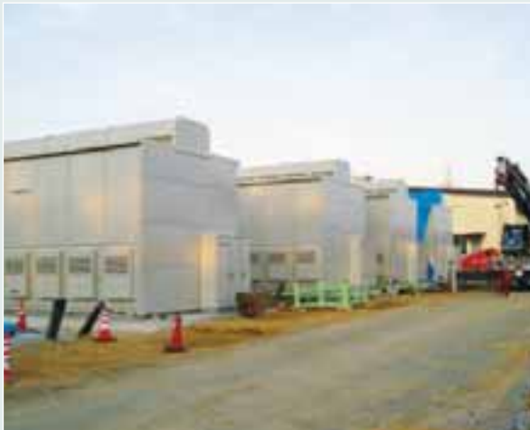
Battery storage system for wind-power generation plant
