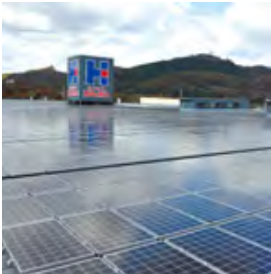
Solar power equipment at a Ninohe Home Center
