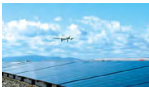
Kansai International Airport generation facility
