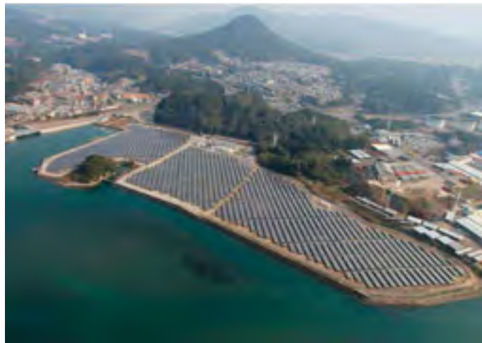
Sasebo megasolar generation facility
