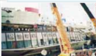
Hankyu Corporation: Earthquake reconstruction work (Hyogo Prefecture) Recovery work on traffic infrastructure destroyed by earthquakes
