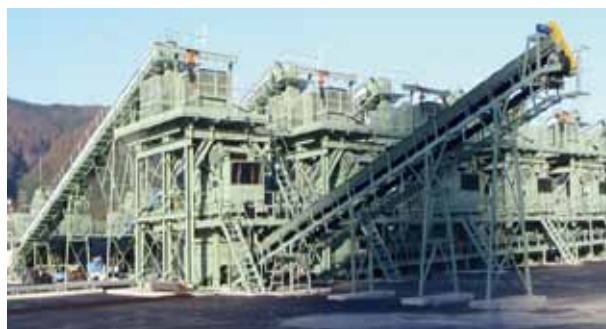
Plant to remove salt from disaster-related waste (Ofunato, Iwate Prefecture)
