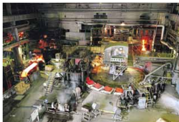
Refining furnace and casting machine
