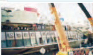
Hankyu Corporation: Earthquake reconstruction work (Hyogo Prefecture) Recovery work on traffic infrastructure destroyed by earthquakes
