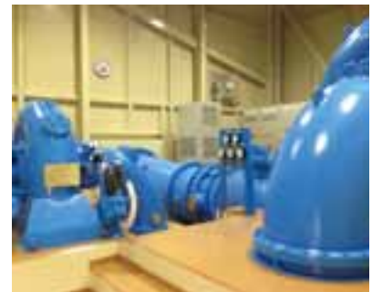
Inawashiro Small Hydropower Plant
