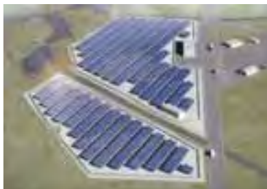
Megasolar power plant in Tsugaruishi district
