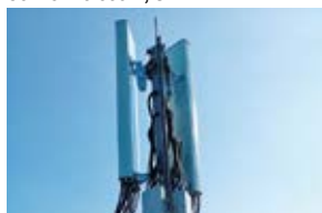
Cellnex Telecom, S.A.
