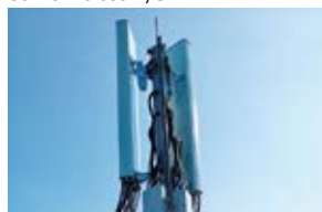
Cellnex Telecom, S.A.
