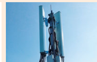
Cellnex Telecom, S.A.
